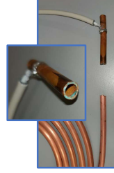
Fig. 13. Corrosion on Current Injector
